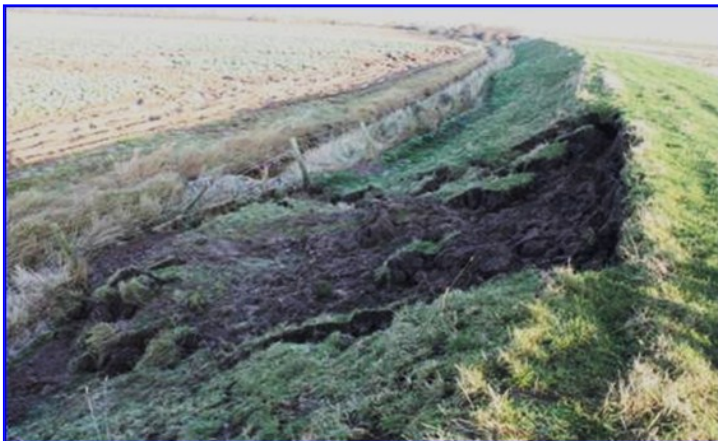
Photo of 2013 overtopping damage to sea banks
